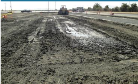
Original 'Bay Mud' Soft Subgrade Caused by High Groundwater
