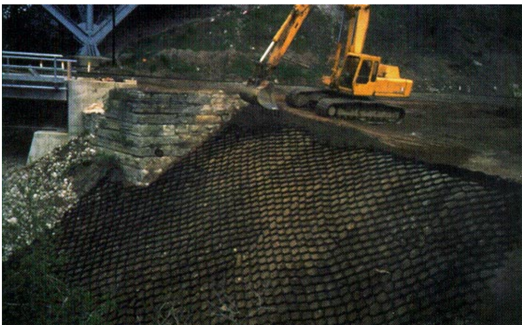
A cellular confinement system with polymeric tendons is used to rehabilitate this 1.5H:1V slope.
