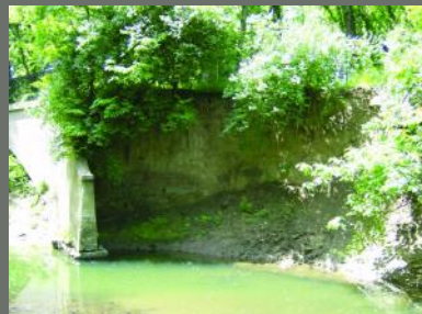
Abutment preconstruction showing erosion and loss of the trail.
