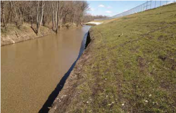
The Geoweb retaining wall protects the toe of the reconstructed levee from erosion by the Little Buck Creek.
